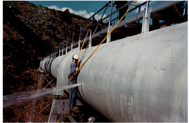
Curtis Wood Repairing a hole in the Willow Creek Siphon circa ~1990's
